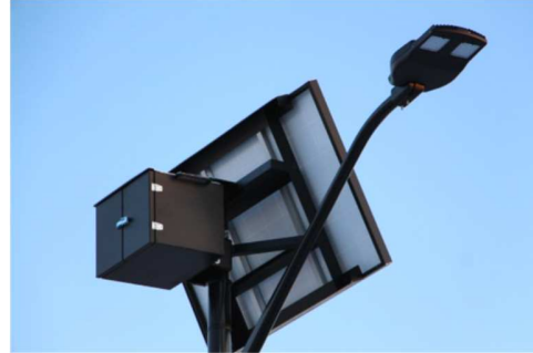
Two 12V batteries are placed in series inside of an insulated battery box.
